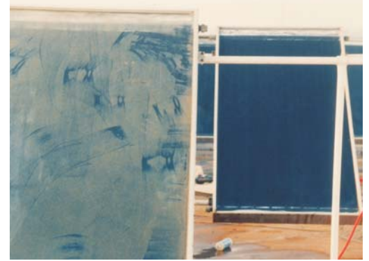
The panels would quickly get dirty due to the dry and dusty climate
