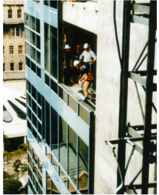
ClearShield was specified to reduce delays during the construction of the Bank of America in Sydney, Australia
